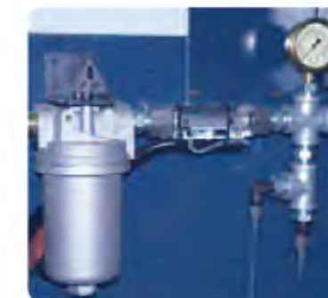
▶▶ Lubrication filtering unit ▶▶ Pressure sensor
